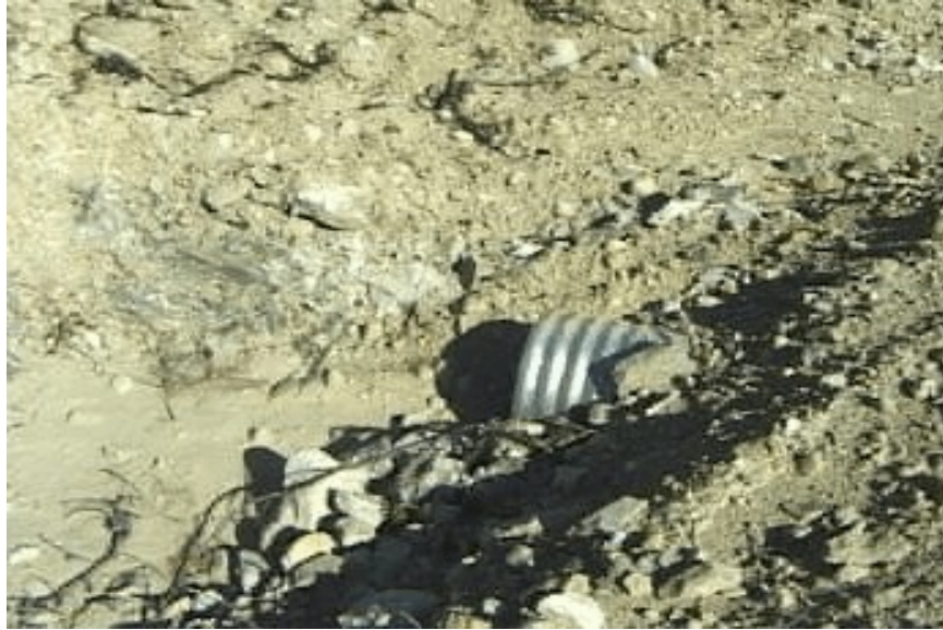
Photo 5 – Partially buried culvert inlet
