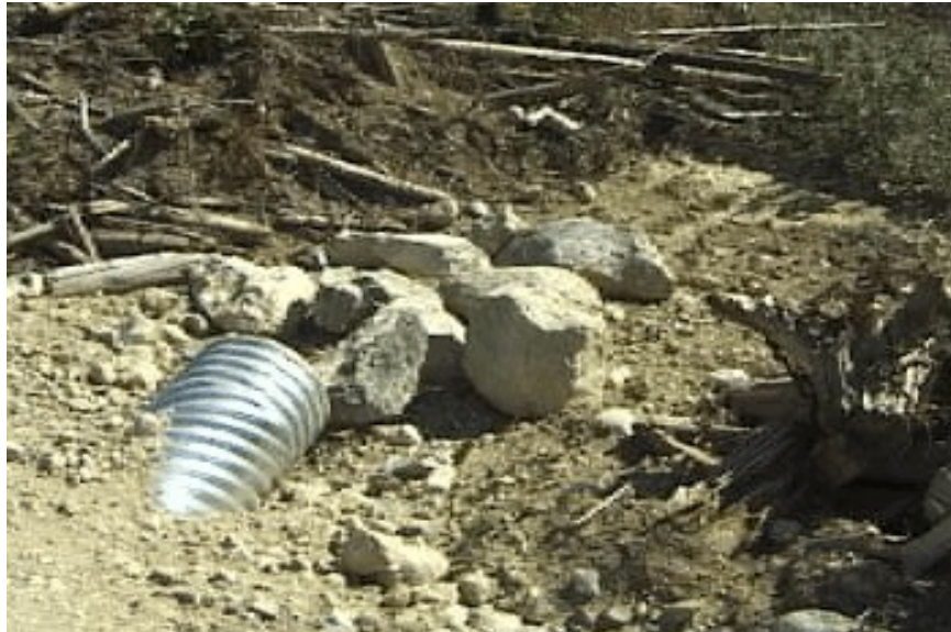
Photo 6 – Rudimentary energy dissipator at culvert outlet
